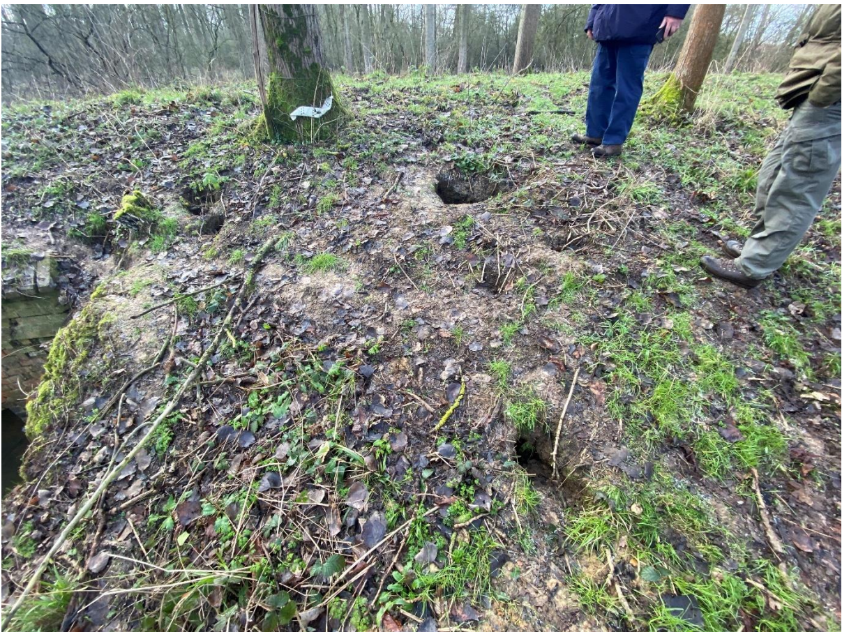
Plate 2 Example of badger burrows in the dam, near to one of the culverts.
