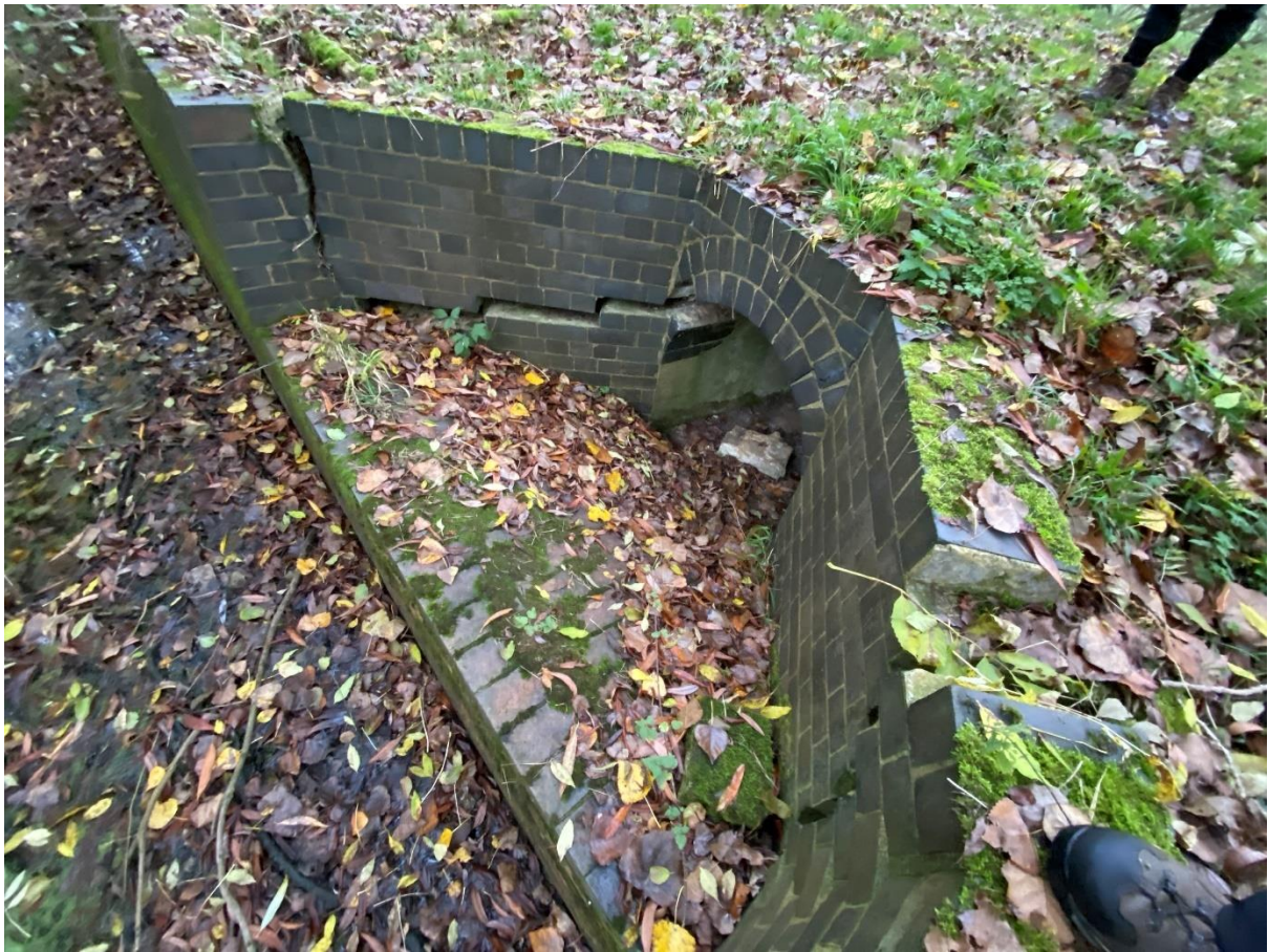
Plate 3 Headwall of one of the culverts shown sunken with broken headwall.
