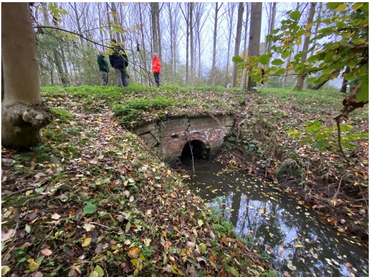
Plate 4 Headwall of second culvert shown broken, Condition of brickwork inside culvert also very poor.
